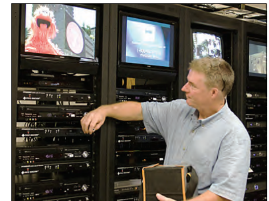
Lee Harding, Video Engineer for WCVE Education, on the job at N.B. Clements Junior High School in Prince George County.
